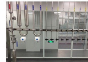
Clean room sewage treatment
