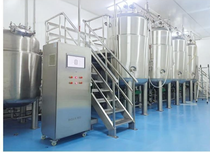
Four-tank inactivation system
