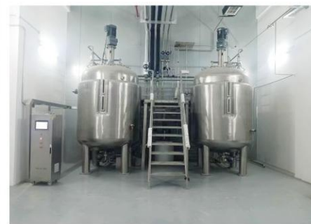
Two-tank inactivation system
